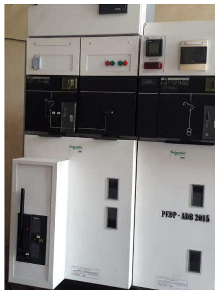
Figure 3. Model cubicle 20 kV
