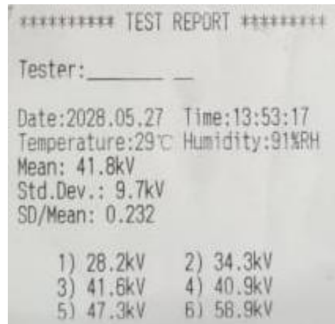
Figure 5. Transformer Oil Test Report Result Data on Distribution Transformer 25 kVA 3 Phase 50 Hz 400 V/ 20 kV - TR. Centrado 25 kVA SN. 1511009
