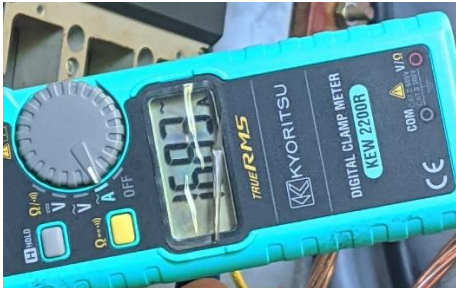
Figure 11. Current measurement on neutral
