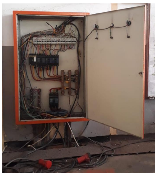
Figure 4. Main Distribution Panel (MDP) Low Voltage (LV) 3 Phase 50 Hz 380/ 220 V 4 x 70 mm 2 as Incoming for power supply Energize Step-Up Distribution Transformer Capacity 25 kVA 3 Phase 50 Hz 400 V/ 20 kV
