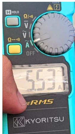
Figure 8. Current measurement on phase R
