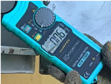
Figure 12. Current measurement at grounding
