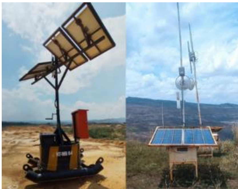
Figure 2. Wi-Fi Access Point as outdoor wireless in BPB
