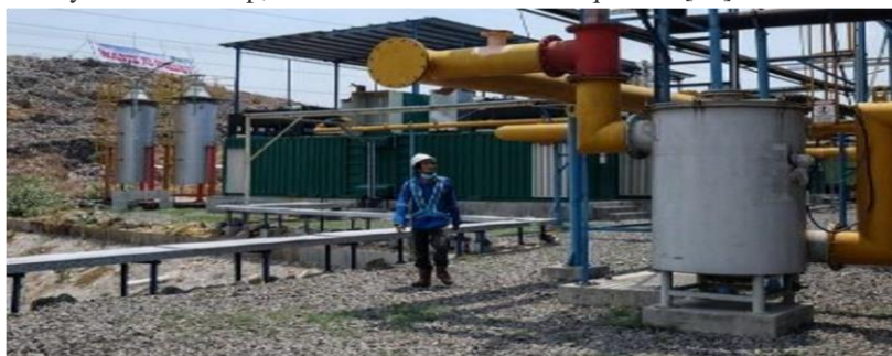
Figure 2. Putri Cempo Solo solar power plant
