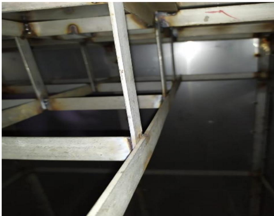
Figure 1. Upper frame design that functions as a removable cover as well as load-bearing.
