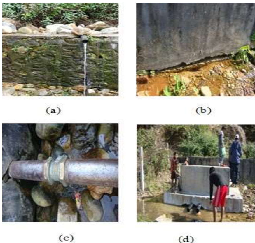
Figure 2: Rusting of cement structures, Corrosion of masonry wall of sump well (a) to (d )
